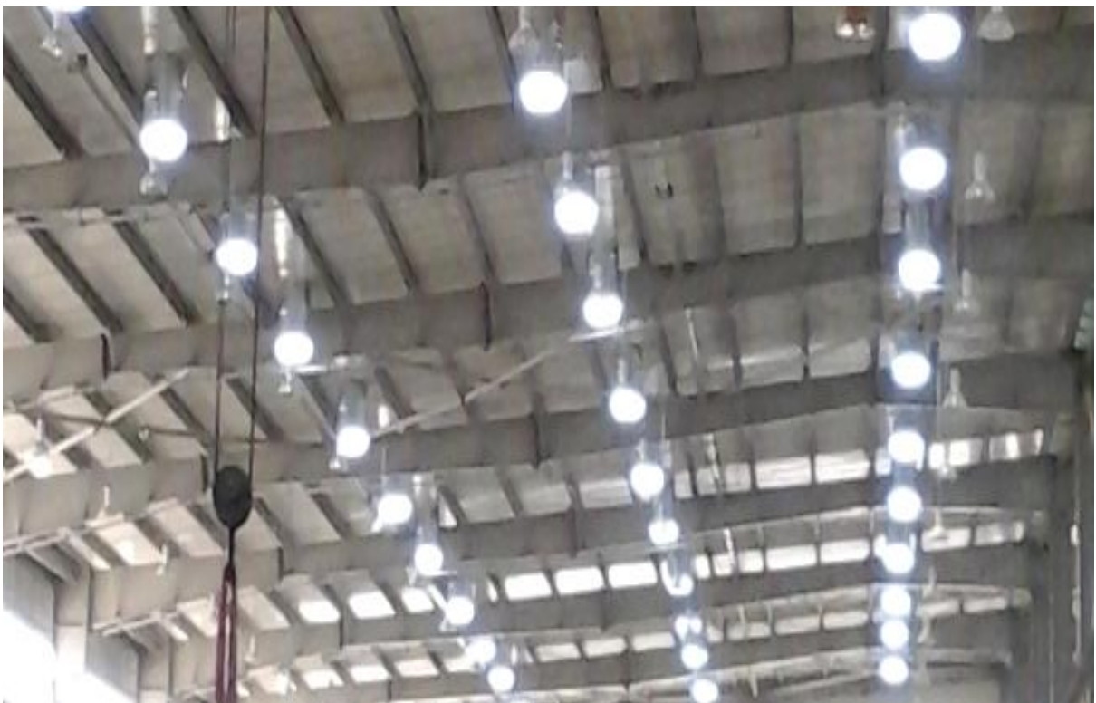
Pipe-Cool Day Light System
