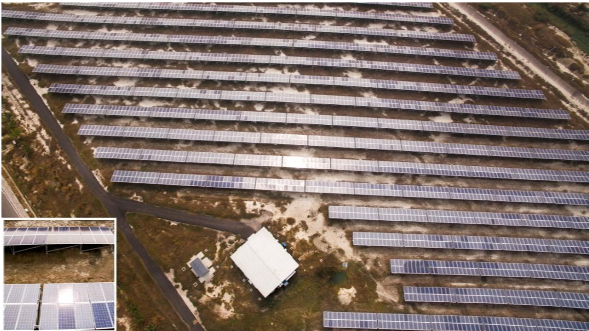
3 MW Solar Power Plant
