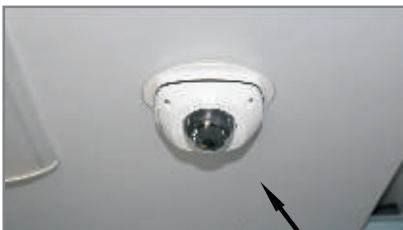
POE (Power Over Ethernet) CCTV Camera
